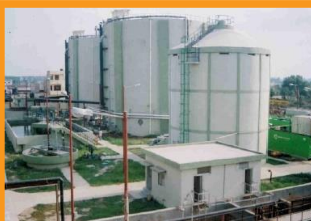
Haibowal Dairy digester tanks and biogas storage unit
