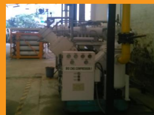
Bio-CNG compressor unit
