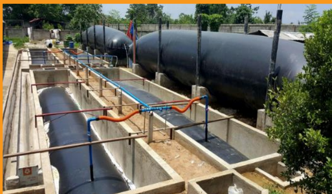
AD System Installed at Bulucan Farm Cooperative
