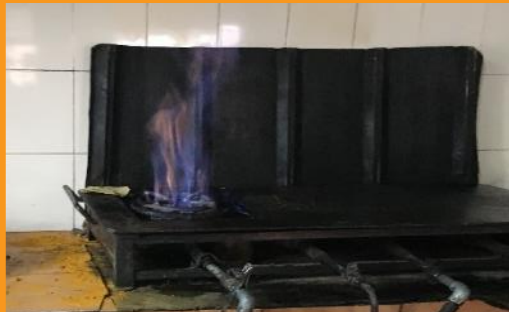
One of the kitchen's biogas powered stoves
