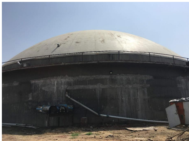
Figure 24. Completely Mixed Digester
