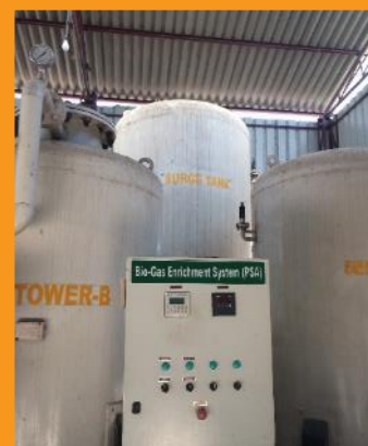
Biogas purification system
